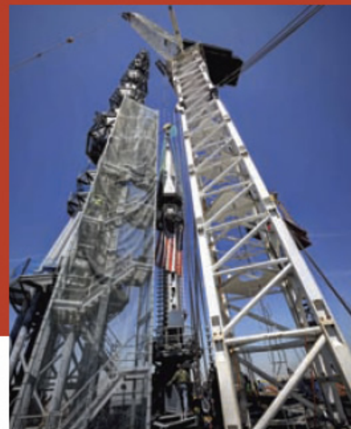
The final spire section was lifted to the roof of the building on May 2 and was erected to its final height on May 10.
